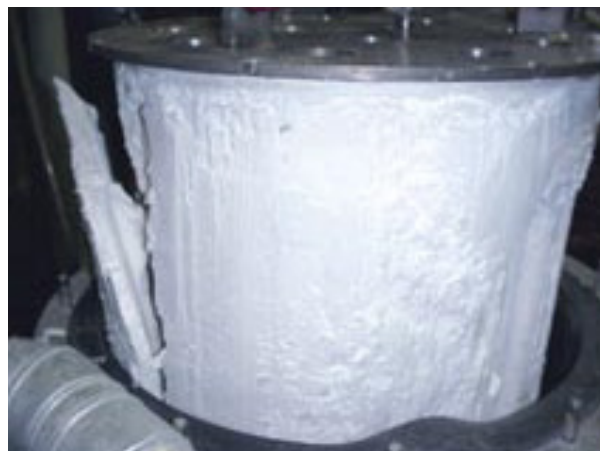
FIGURE 11. A MULTIPLE-CARTRIDGE DUST FILTER, COMPLETELY BLOCKED BY SOLIDS
