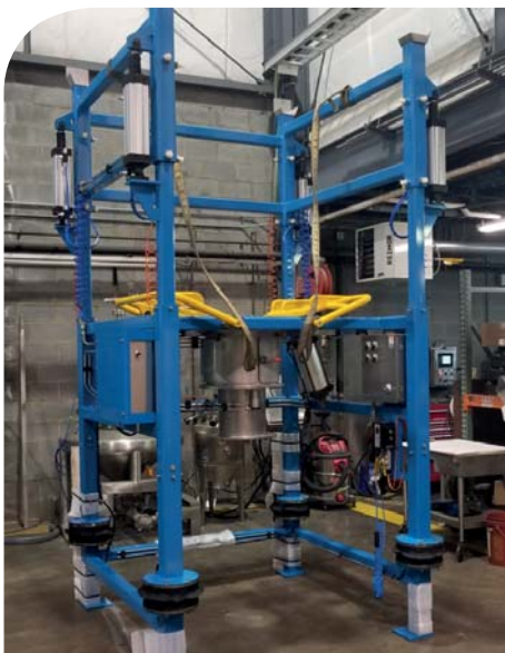
Bulk bag unloading station
