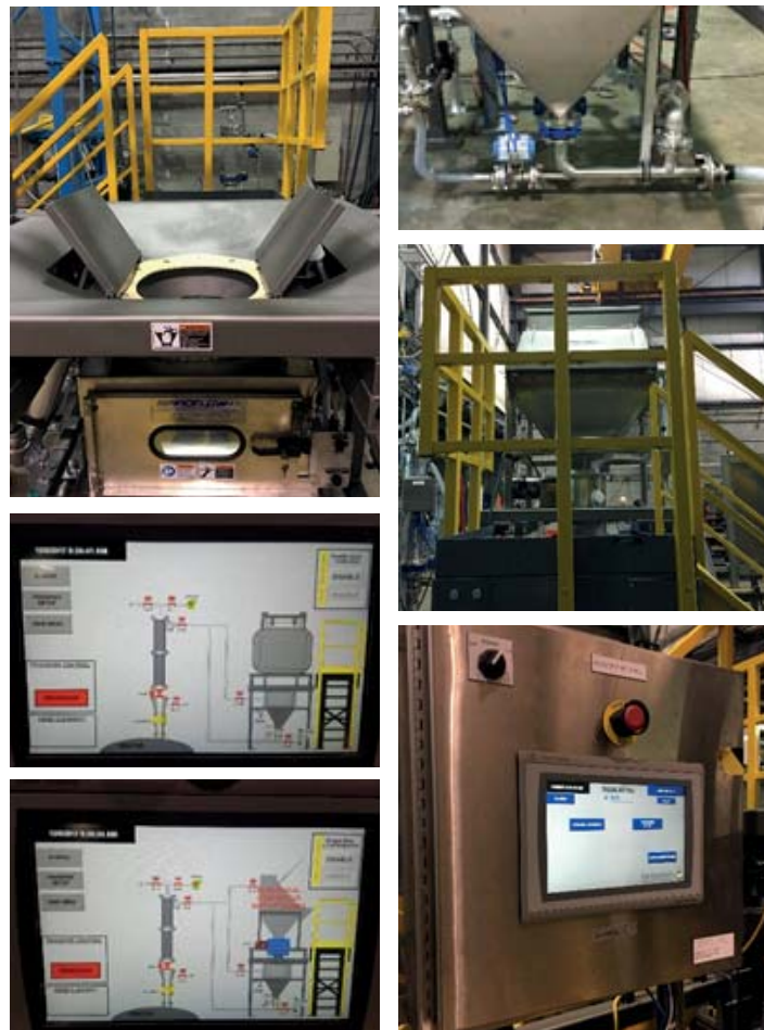
Screenshot samples of PLC & HMI controls display.
