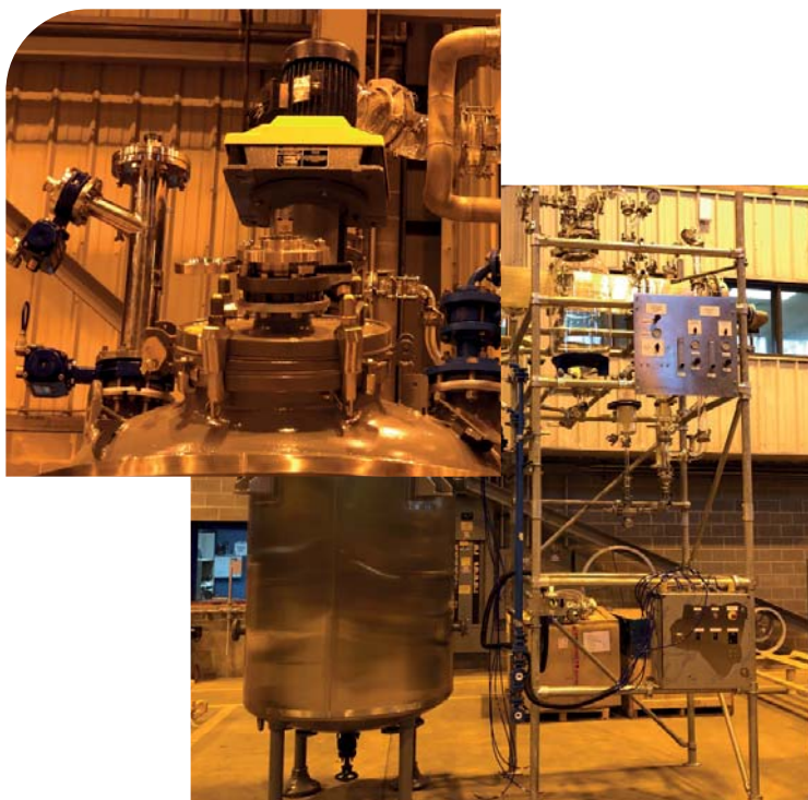
Powder Pump system installed on reactor / Glass overheads and control panels
